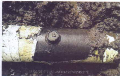
Pipeline exposed showing nipple installed
